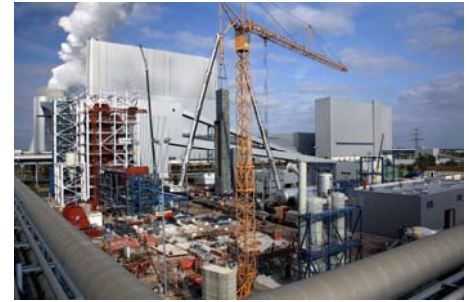
Construction of the Vattenfall 30MW oxy-fuel pilot plant in Schwarze Pumpe, Germany
